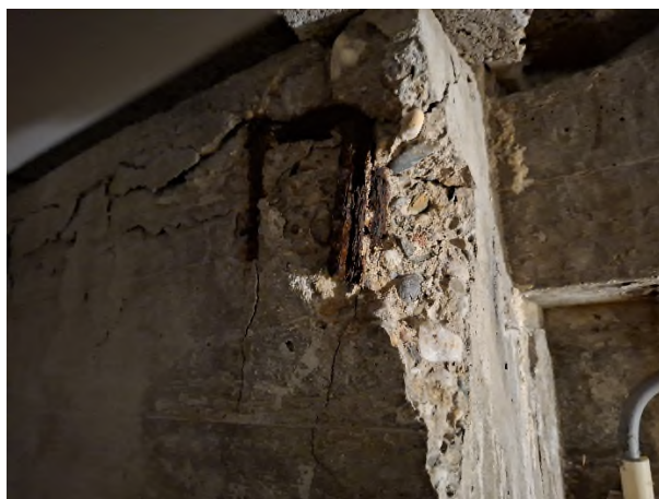
Afb. 1 – Chlorideschade beton bassin
