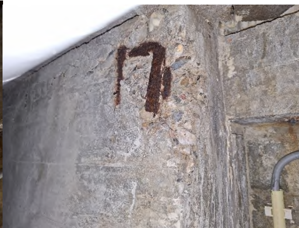
Afb. 2 – Chlorideschade beton bassin
